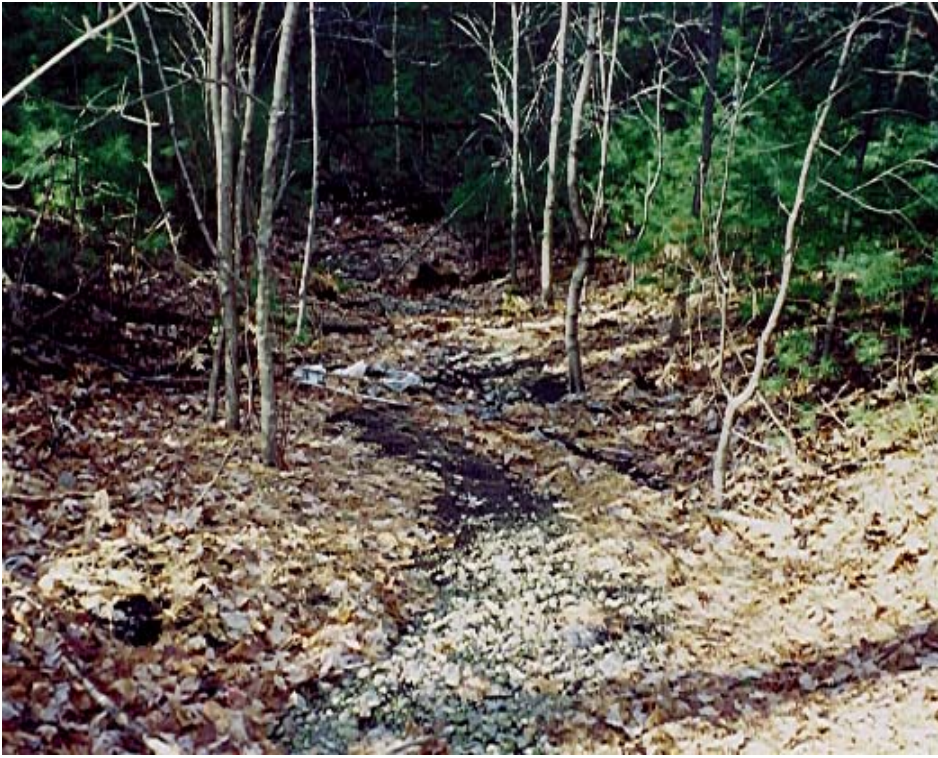
Figure 3-4. View of the Scoured Swale that Enters the Detention Pond from One Watersedge Drive Discharge.
