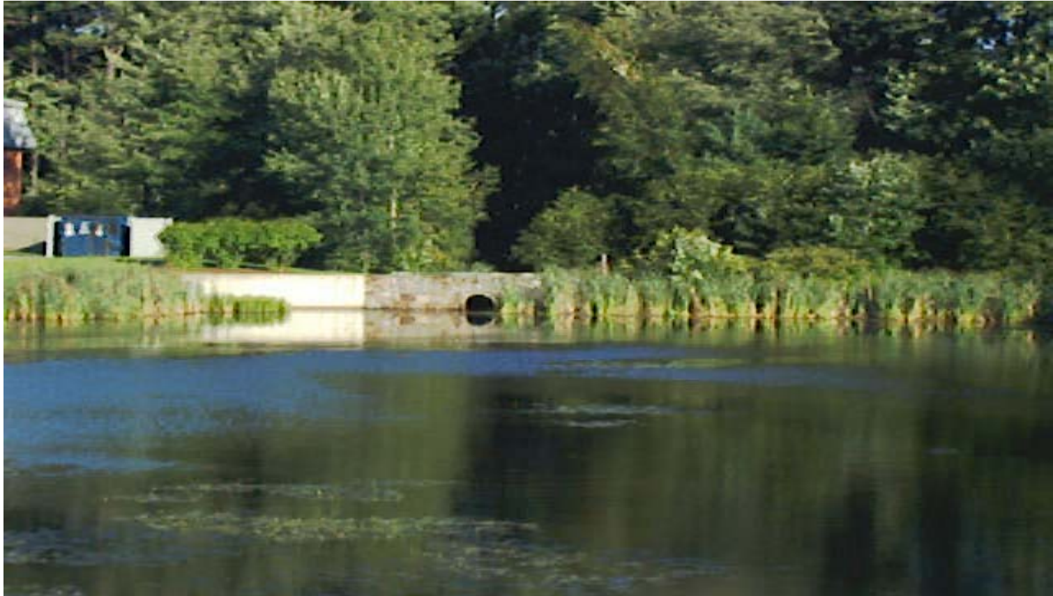
Figure 2-7. View of the Detention Pond from Blackstone Drive Showing the Outlet. This Marks the Beginning of the Unnamed Brook Entering Holt Pond.
