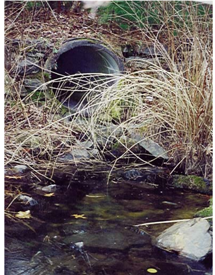
Figure 3-5. View of Second Watersedge Drive Discharge into Detention Pond. The Swale Area Immediately Below is Scoured.
