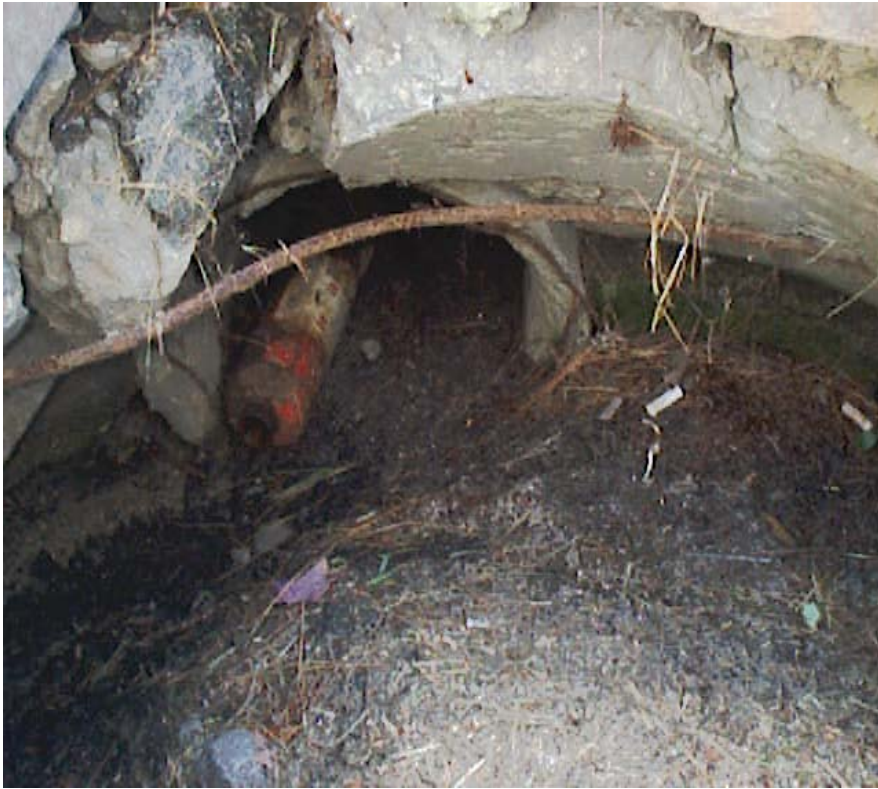
Figure 3-9. Thorton Road Catch Basin Full of Sediment and in Need of Maintenance.
