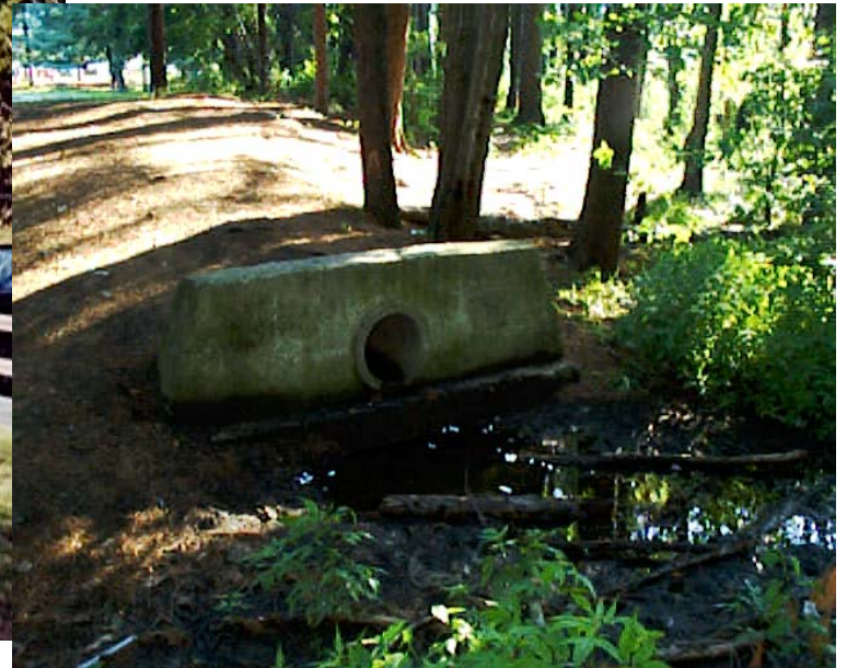
Figure 2-6. View of Direct Discharge to Unnamed Brook Entering Holt Pond.
