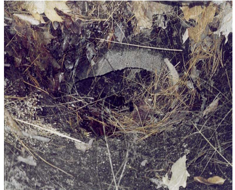
Figure 3-10. Clogged Discharge Near Larchen Lane. Sediment has Built Up Around the Pipe such that It is Actually Below Grade.
