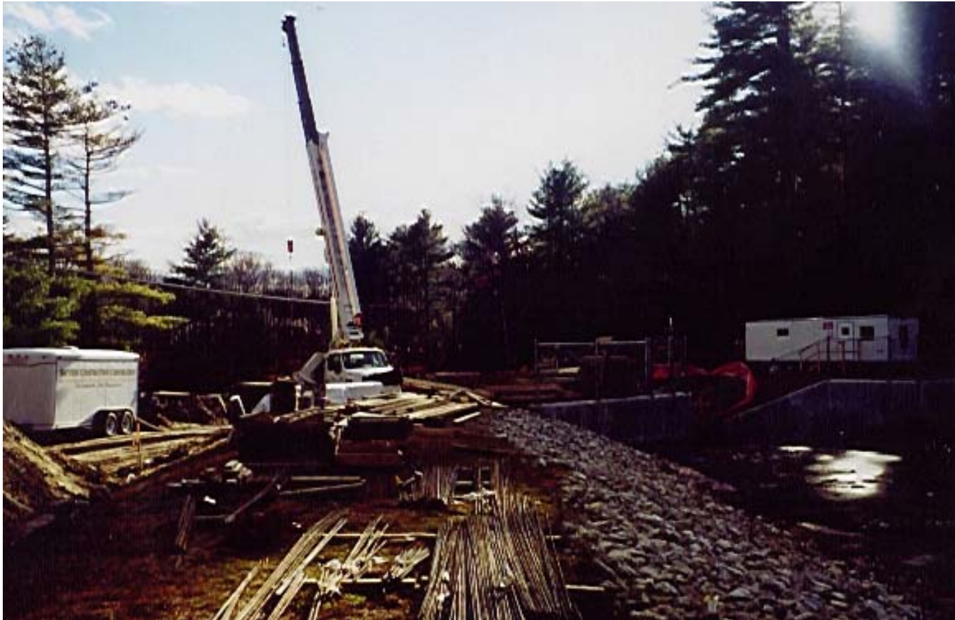
Figure 3-12. Construction of a New Bridge on Thorton Road. The New Construction Incorporates a Swale System that Handles the Runoff From Thorton Road.
