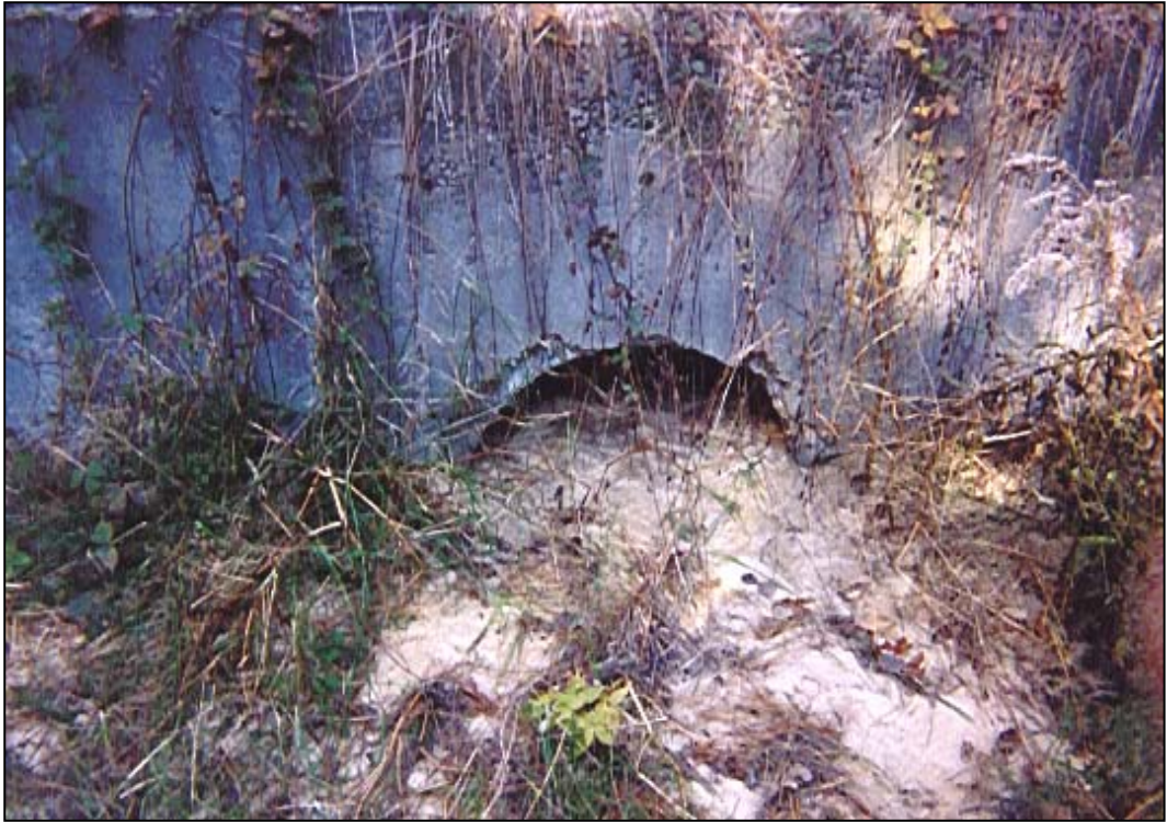
Figure 2-16. Cornerstone Discharge Blockage
